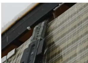
Fig. 1.2. Inappropriate support studs
